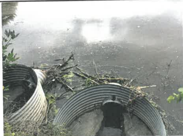
Accumulated debris at outfall structure
