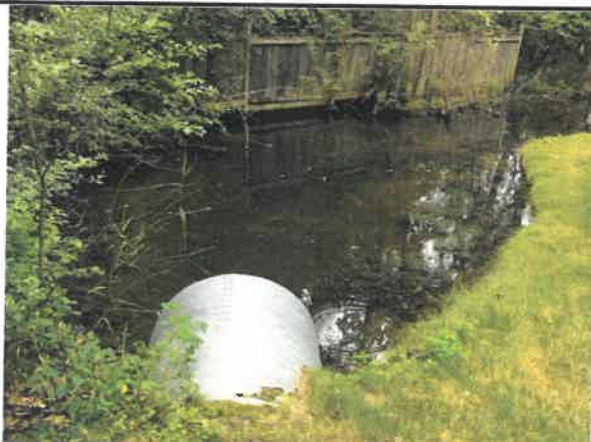
Easterly view of outfall structure looking westerly at release side of structure
