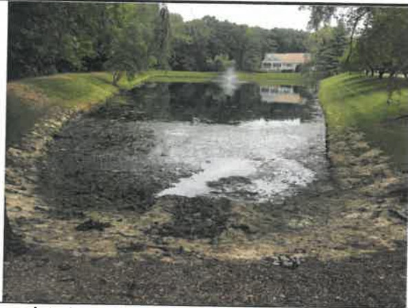
Accumulated sediment/ debris in storm inlet pipes on southerly side of basin
