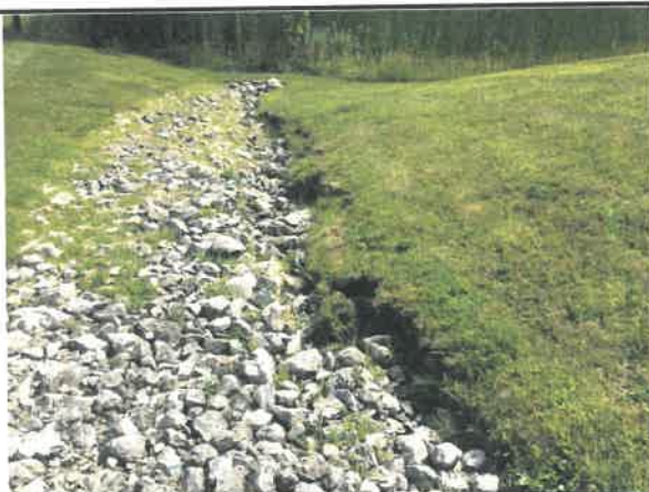
Side of trench eroding away
