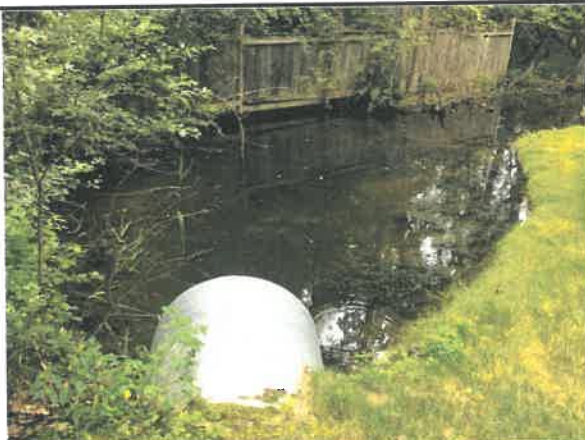
Easterly view of outfall structure looking westerly at release side of structure
